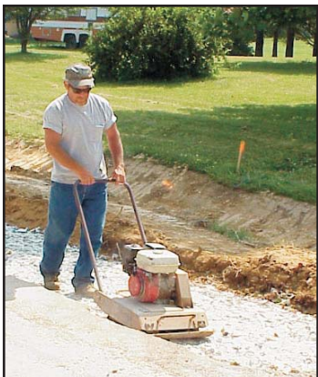
A Henderson County Road Department employee uses a hand compactor to level a four-inch-thick layer of PGA in a five-foot-wide trench as part of a road-widening project in June. Henderson was the first county in Kentucky to use pulverized glass aggregate as fill in a road project.
