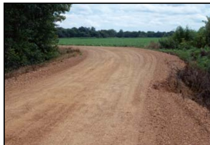
The sharp curve in this road at the Wildlife Refuge will be straightened and a new bridge will replace the culvert.
