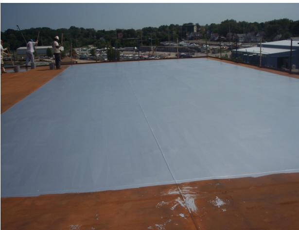
FIGURE 14: Rust Grip® Applied to Deck of Largest Casino Ship in United States, Michigan City, IN
