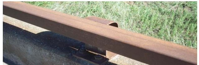
FIGURE 7: Railings Before Rust Grip® 2005, OKDOT
