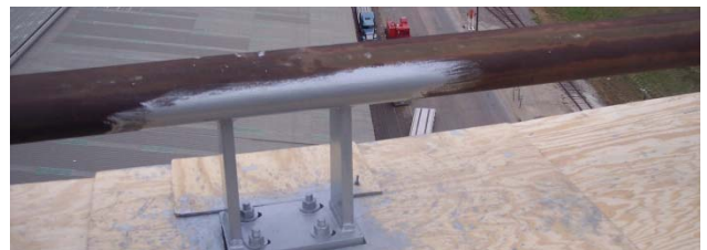
FIGURE 9: Railings Before Rust Grip® 2006, TXDOT
