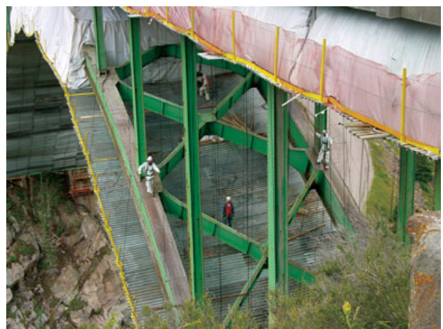
FIGURE 2: During the paint removal process, workers enclose the work area in vacuum-sealed tarps to contain and collect lead-based paint debris for offsite disposal.
